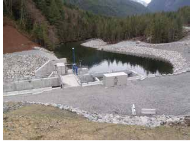
Diversion System Hydraulic Structures Pictured Below
